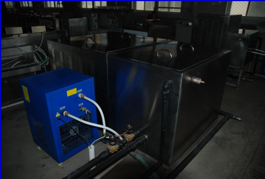
Machine for cooling water(Automatically)
