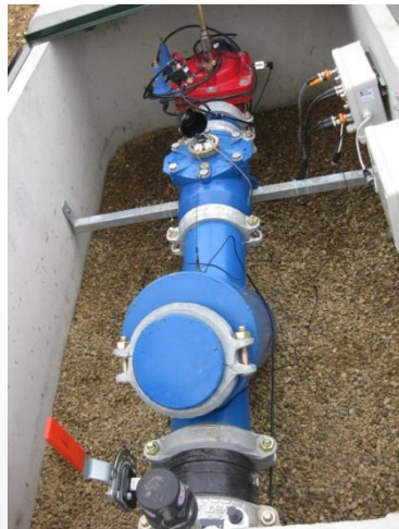
Hydrant in the field
